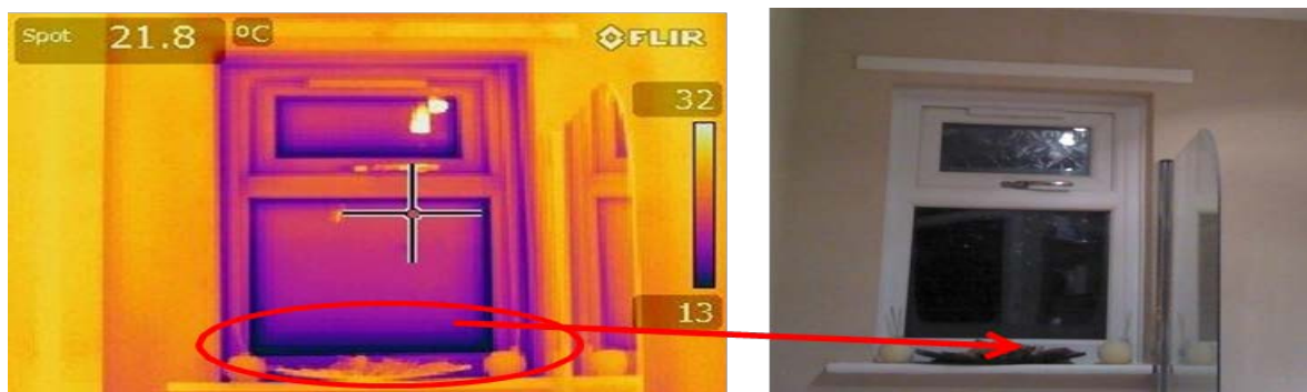
Figure 21: Detections around windows at the bottom.
