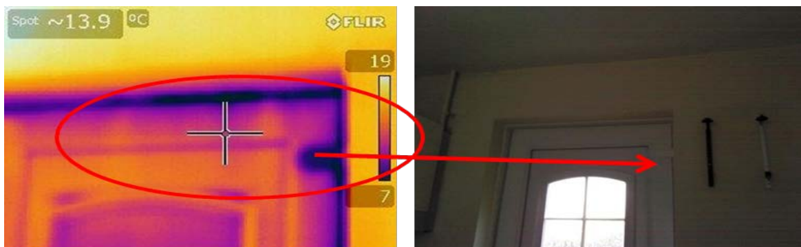
Figure 20: Defective seals on the top of the door profile
