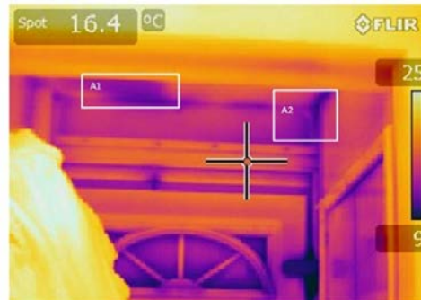
Figure 1: The air leakage defects
