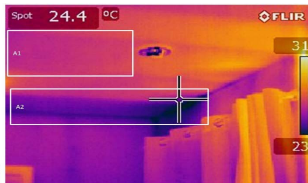
Figure 2: Missing insulation defects
