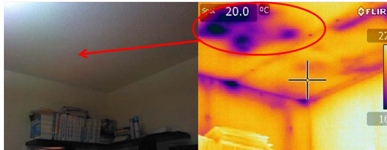
Figure 11: Wide spot of air infiltration due to missing fitted insulation in the loft
